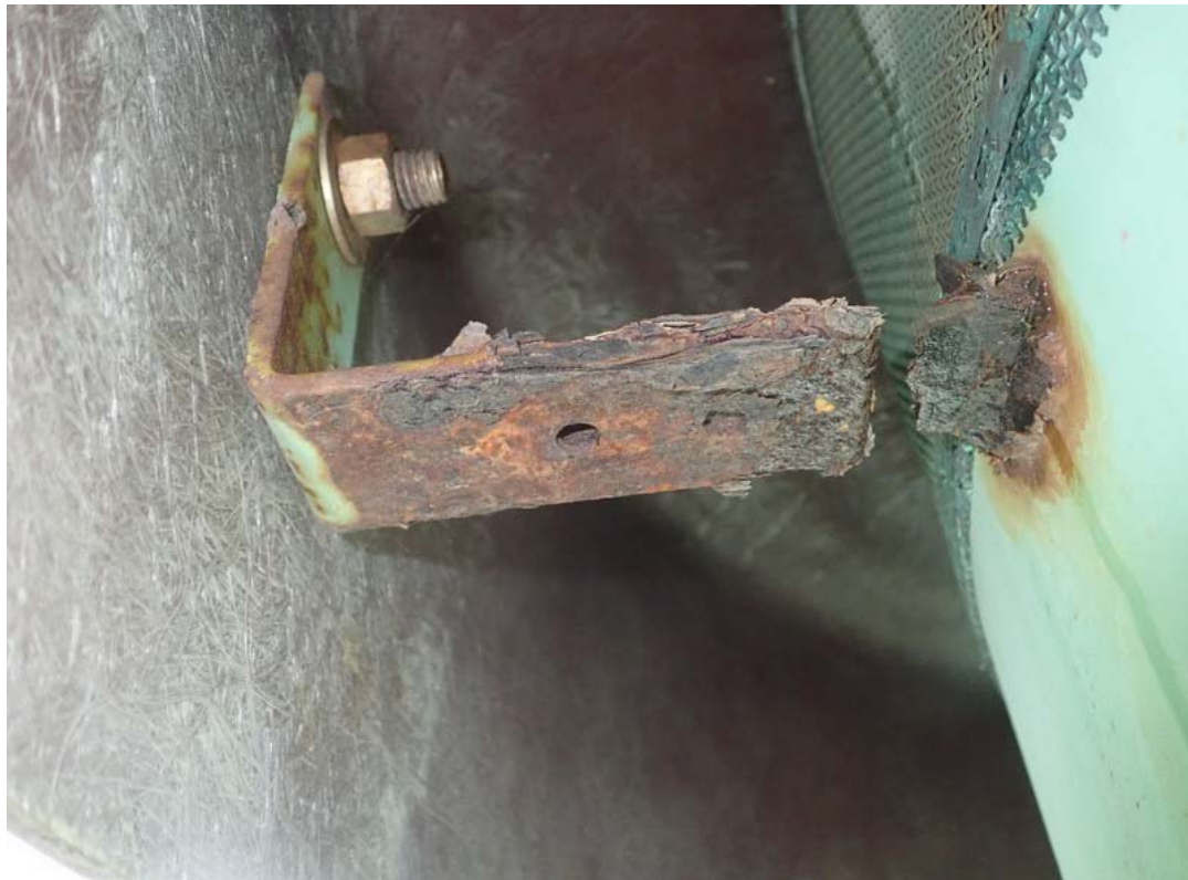
This is a view of the underside of the vent hood. The screen appears to be intact and bug proof. Serious corrosion has damaged the roof vent hood attachment that keeps the hood from blowing off during high winds.
