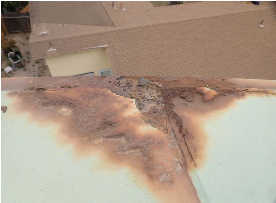
This is an addition view of a typical corroded area on the tank roof.
