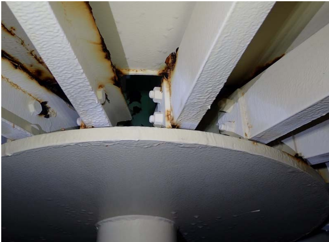
Close view of the center support and rafters. Significant corrosion and heavy staining is visible at the ends of the rafters and at inaccessible areas.
