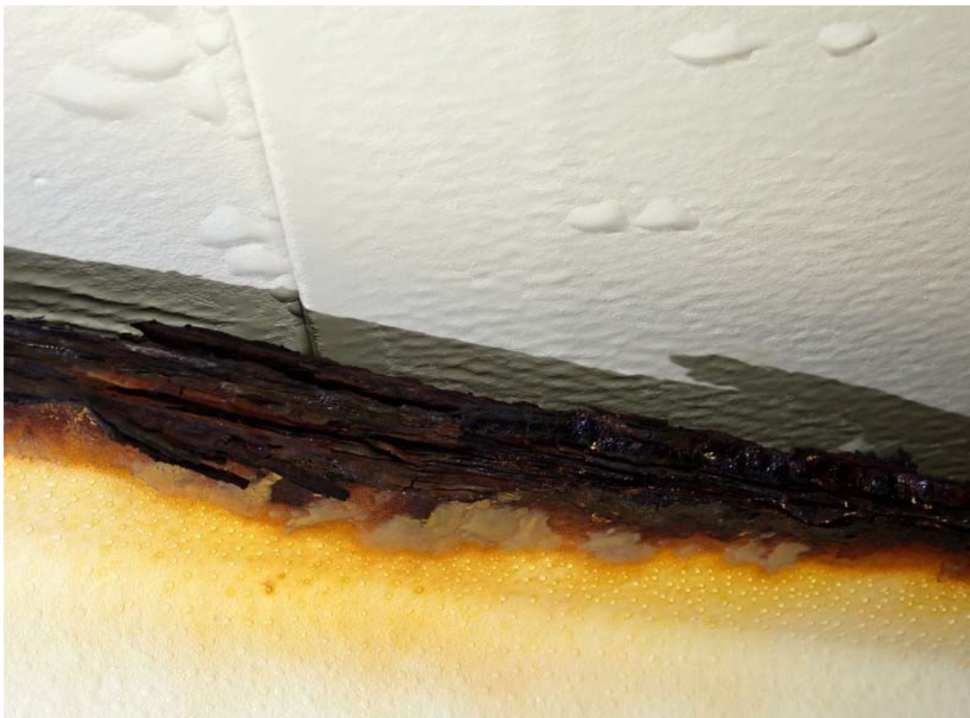
This is a close view of the top flange of a rafter at one of the numerous areas with serious corrosion. This rafter flange has serious metal loss that affect the load carrying capacity.
