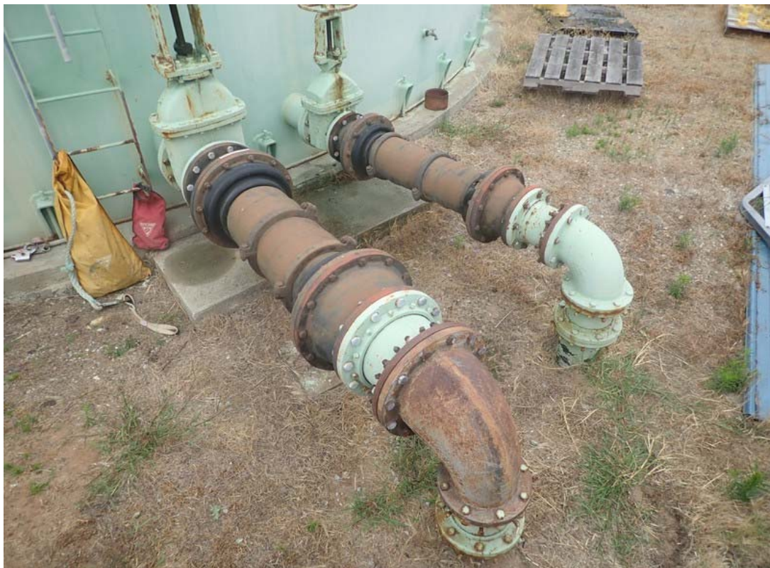
This view shows exterior piping with some corrosion with what appears to be insignificant metal loss. Flexible couplings are in place for seismic movement.
