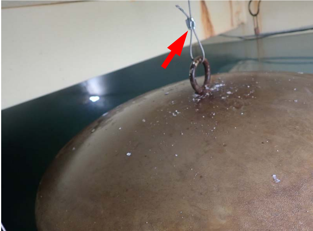
Level gauge float with temporary repair to the attachment. The interior float is not designed for the amount of movement that is created by the adjacent high inlet.
