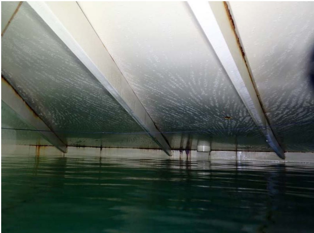
Existing inlet and only a few inches of freeboard.
