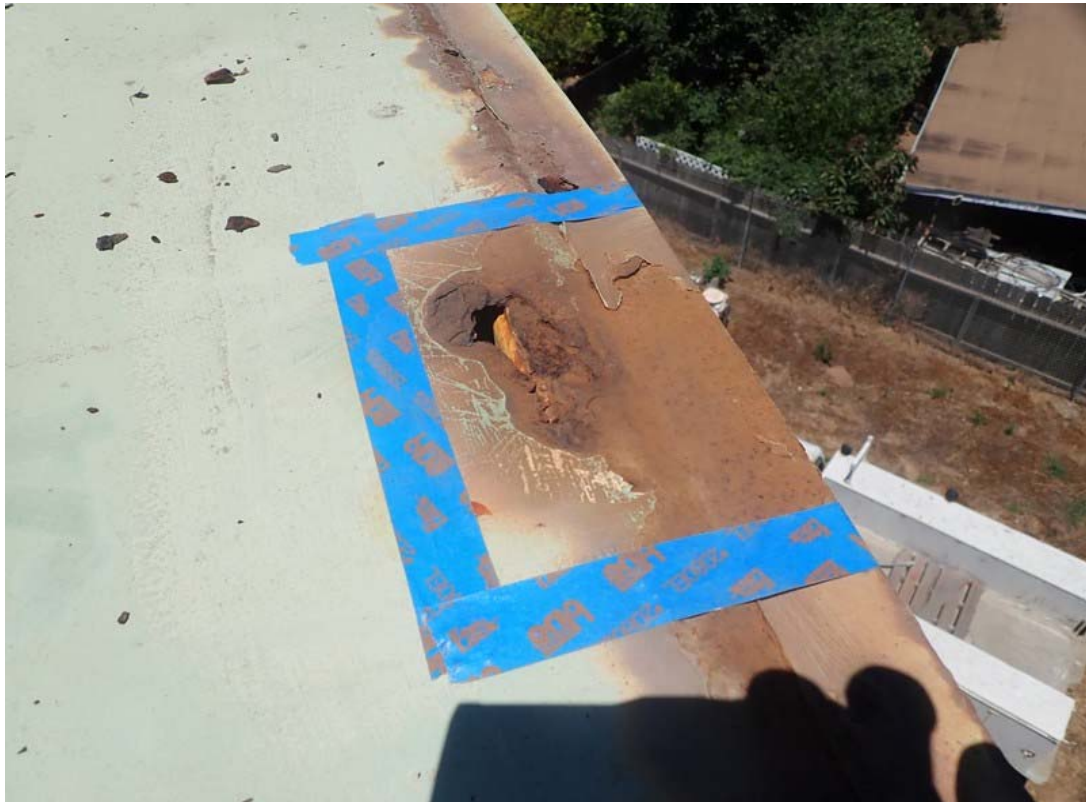
This is one of 10 holes in the roof where ATS provided temporary repairs to immediately seal the roof and meet regulatory requirements.
