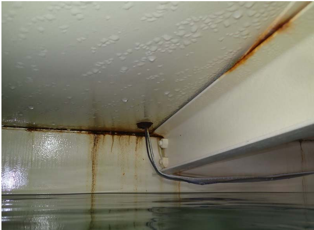
This view is representative of the conditions found on the interior shell, roof plate and rafter.
