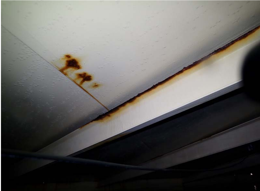
Roof plate rafter with visible corrosion.
