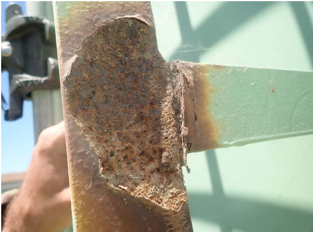
This is a close view of the ladder area shown above. Approximately 50% of the ladder stringer metal thickness is lost to corrosion.
