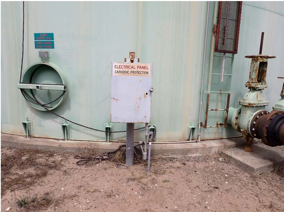
Existing cathodic protection panel. The panel and post are to be removed. The wires shall be removed to the first junction box. The conduit shall be capped and abandoned in place.
