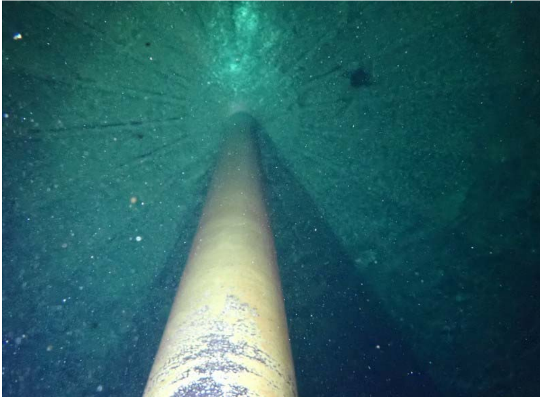
This shot was taken looking upward at the center column. All coatings on the column were in fair condition and no significant corrosion was present.
