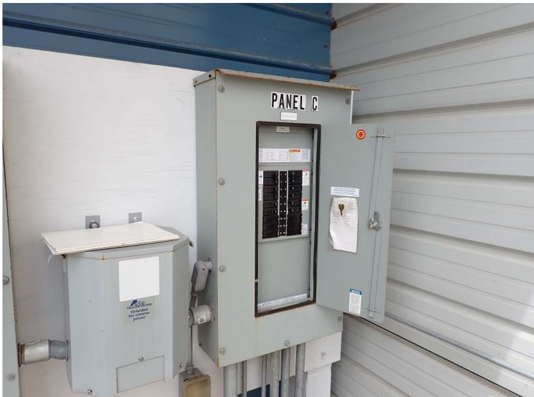
The circuit breaker for the cathodic protection system is in this panel. Other items are on the same breaker.
