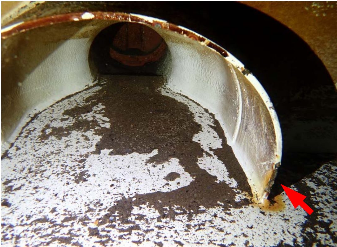
This view shows the interior of the drain pipe. Some corrosion is visible on the interior edge of the pipe (arrow).
