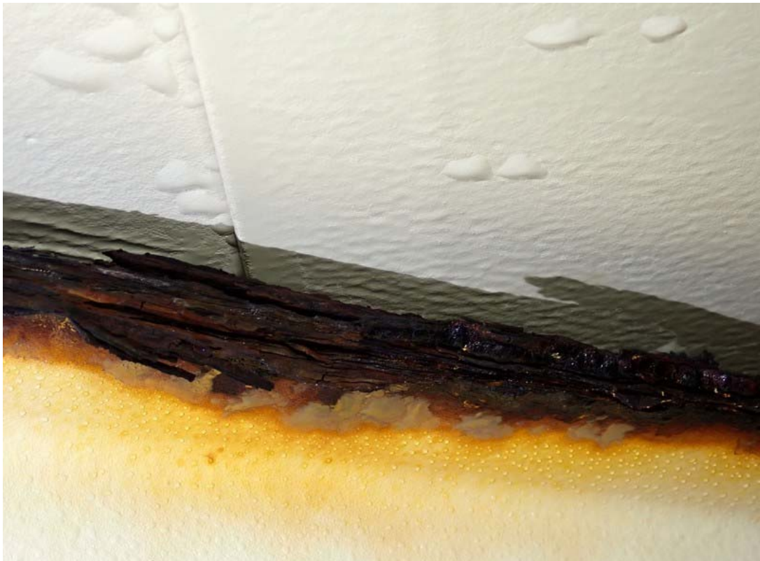
This is a close view of the top flange of a rafter at one of the numerous areas with serious corrosion. This rafter flange has serious metal loss that affect the load carrying capacity.
