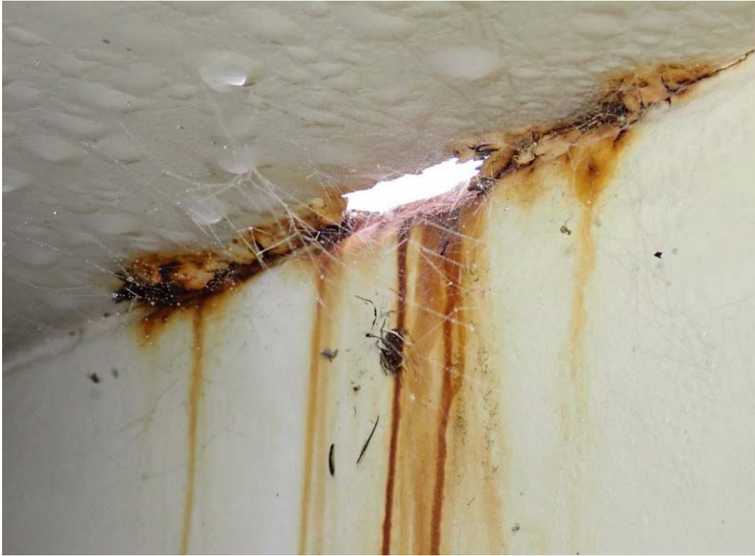
This photo shows a corrosion spot at the interior side of the shell to roof joint. ATS installed a temporary repair to seal this hole. This was the largest hole in the roof but many other locations of serious corrosion are present.
