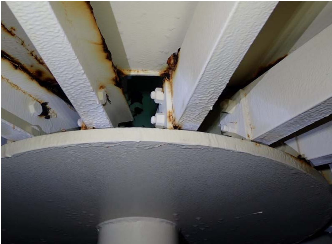
Close view of the center support and rafters. Significant corrosion and heavy staining is visible at the ends of the rafters and at inaccessible areas.
