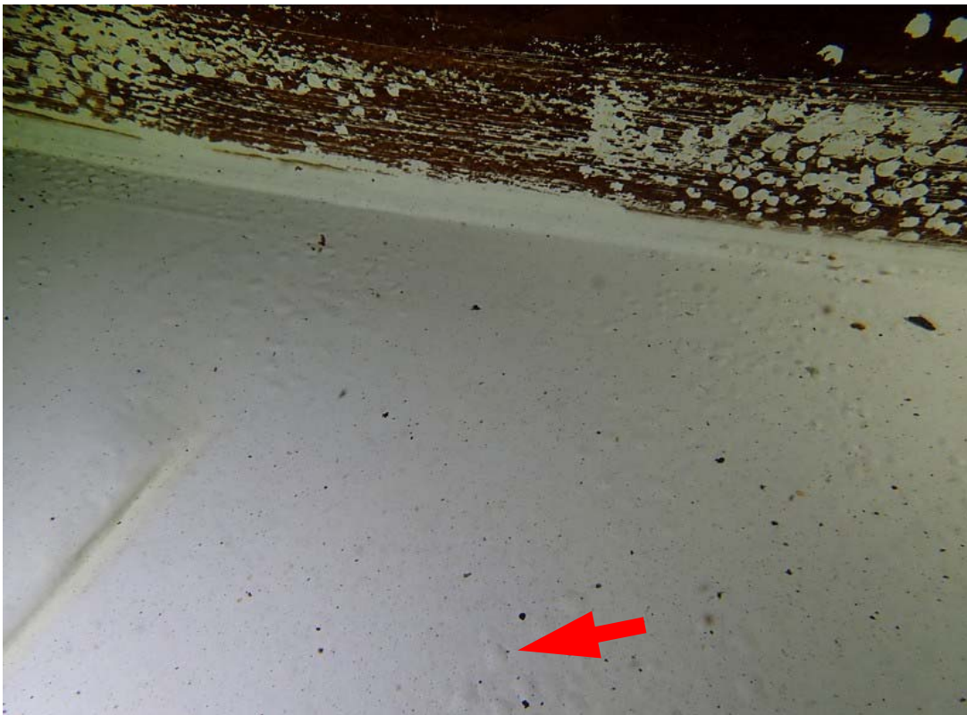
This photo provides a close view of the area shown in the top photo this page. Some scattered blistering is visible (arrow) but no significant corrosion is present.
