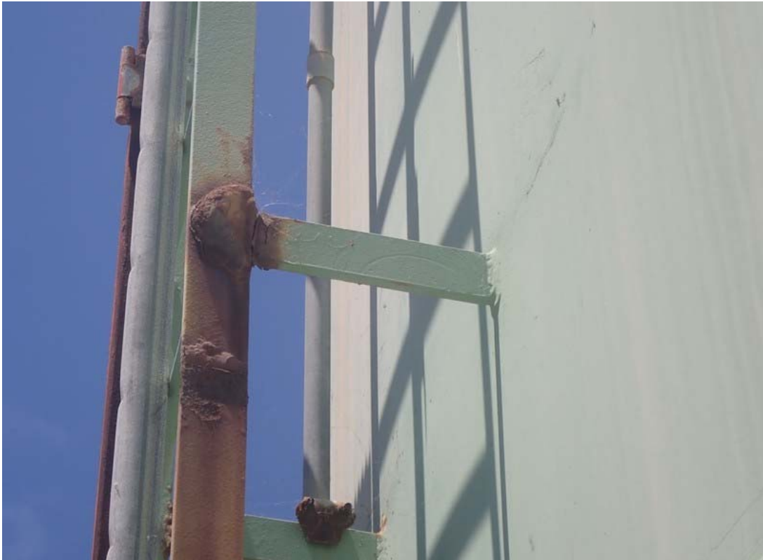
This photo shows one of several areas of serious corrosion on the exterior ladder.
