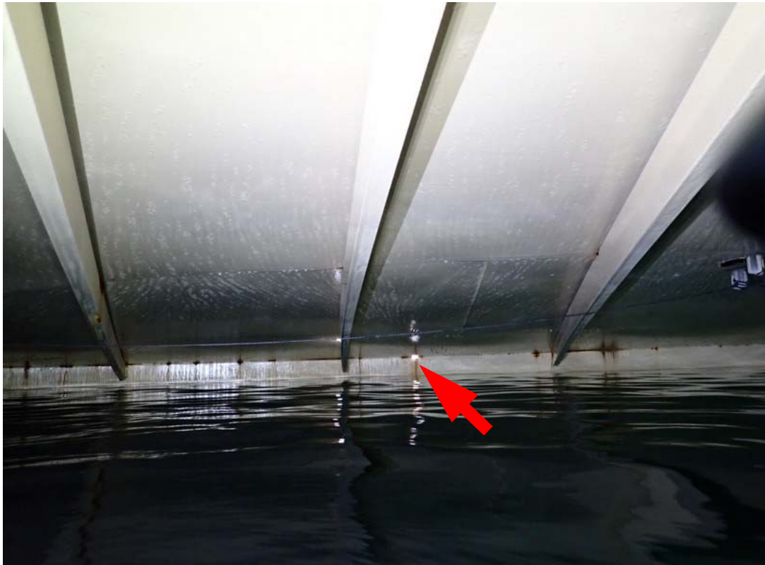
Interior roof plate and rafters. Broad view. Some minor bowing is present in the rafters. This view shows an example of nearly rust free plate but a hole is visible at the shell to roof joint (arrow). The hole was sealed by ATS.
