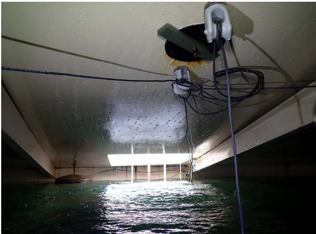
Existing cathodic protection system shall be removed as part of the work.
