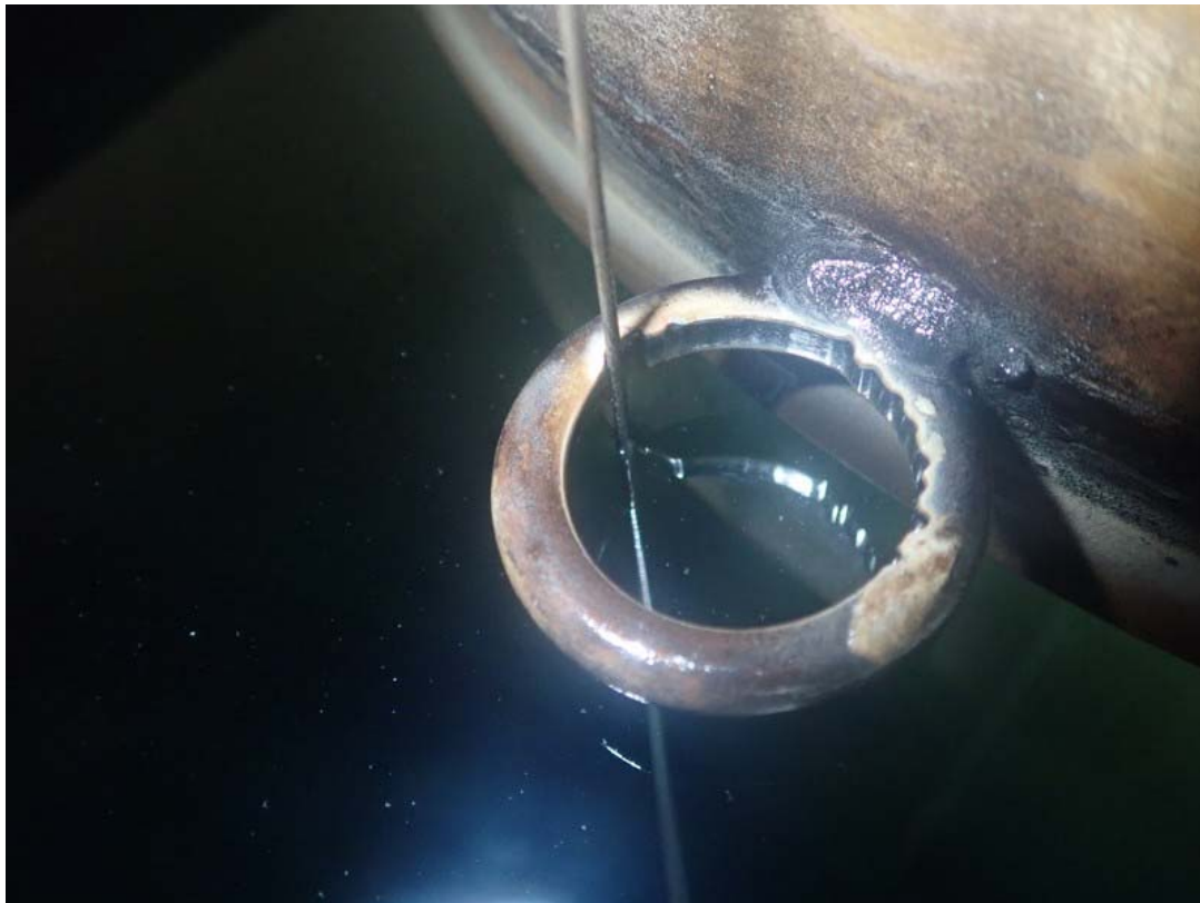
This photo shows the existing level gauge float and guy wire. Wear is visible from wave action produced by inlet flow. A stilling well will be provided as part of this work.
