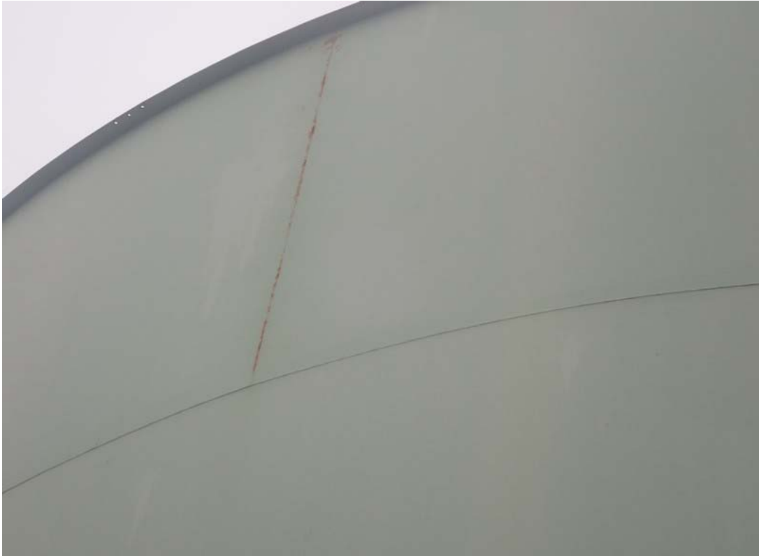
The upper shell and roof joint are shown in this photo. The coatings are in fair condition with significant aging of the coating and scattered corrosion.
