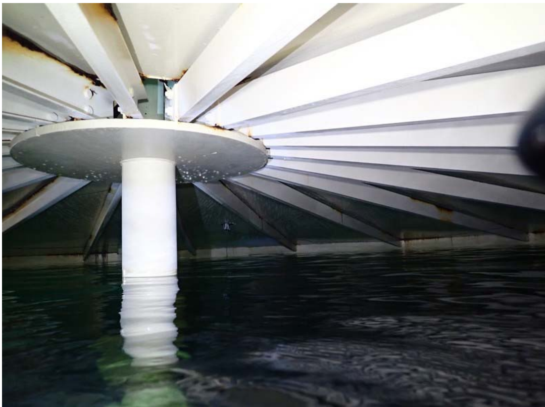
Existing roof column, roof structure and plate that are to be replaced with new formed plate roof.
