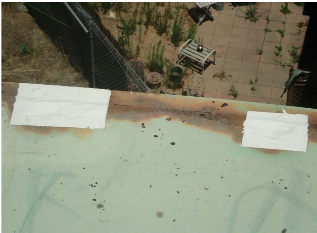
This view shows 2 locations after temporary repair of the holes using fiber reinforced epoxy. The epoxy is NSF 61 certified for use and contact with potable water.
