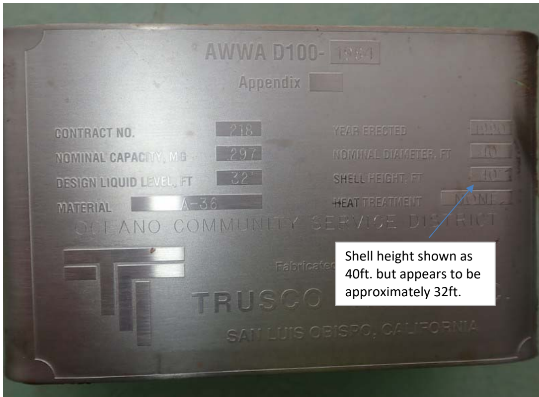
Tank nameplate. The stated shell height of 40 ft. appears to be incorrect. The design liquid level of 32 ft. gives a volume of 0.3 MG so there may be an error there too.
