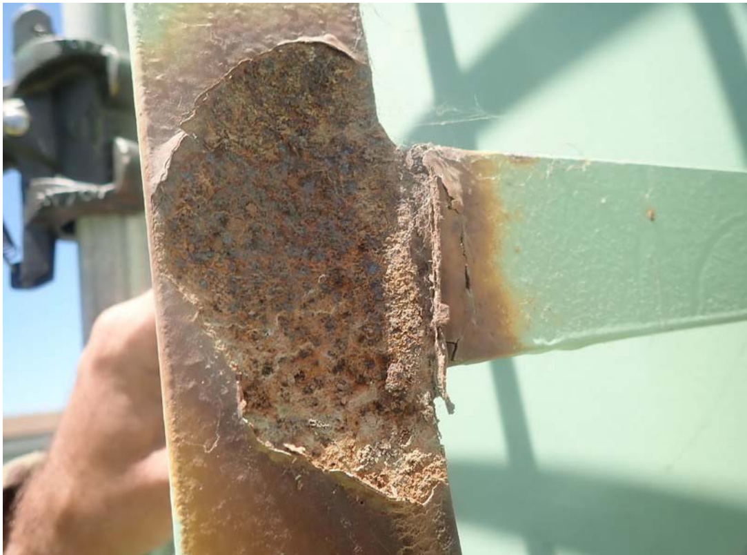
This is a close view of the ladder area shown above. Approximately 50% of the ladder stringer metal thickness is lost to corrosion.
