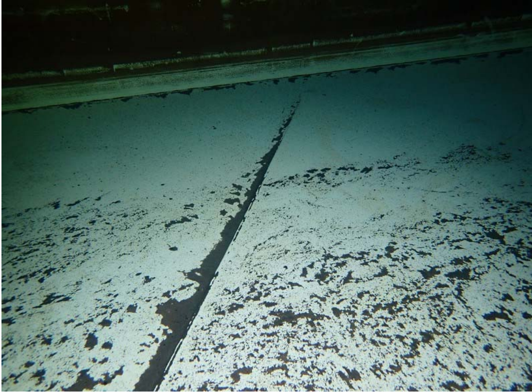
Photo of the interior bottom shell and shell coupling shows the typical condition found. No significant corrosion was noted.
