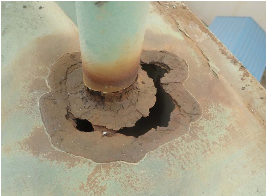
This photo shows serious corrosion and a hole at the base of a guardrail post. This guardrail was designed to help provide safe access to the roof but clearly it is severely weakened.
