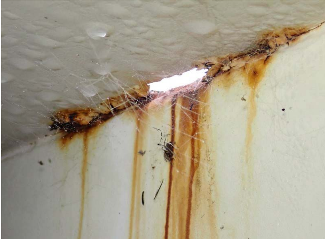
This photo shows a corrosion spot at the interior side of the shell to roof joint. ATS installed a temporary repair to seal this hole. This was the largest hole in the roof but many other locations of serious corrosion are present.
